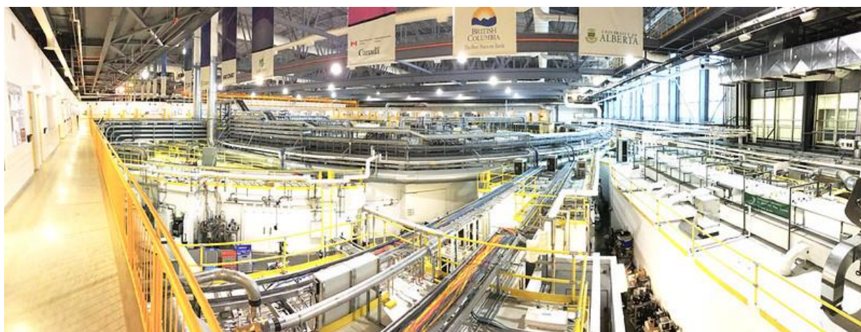
Figure 5-1: Inside the Canadian Light Source Facility | Flickr 1 (Source: CLSI)
